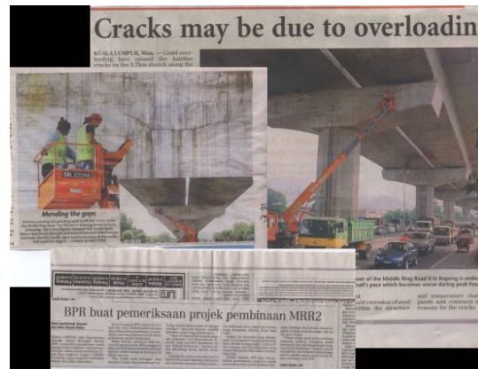
a) Cracks at the pier heads of MRR2 flyover
