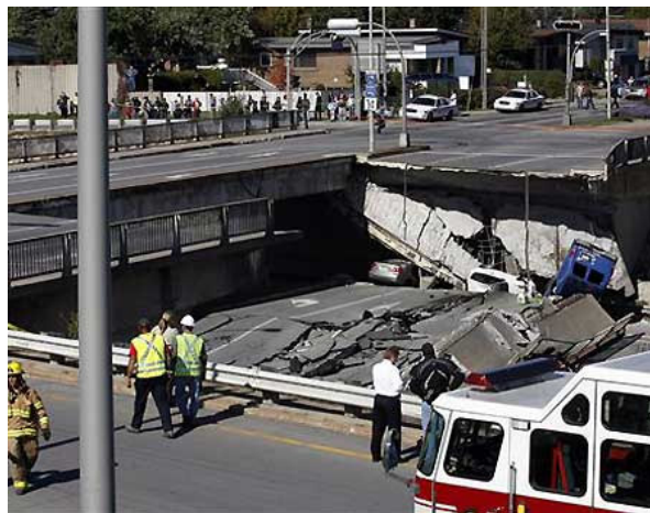
Fig. 2 Overpass collapse at Laval, Canada [from the Internet]
