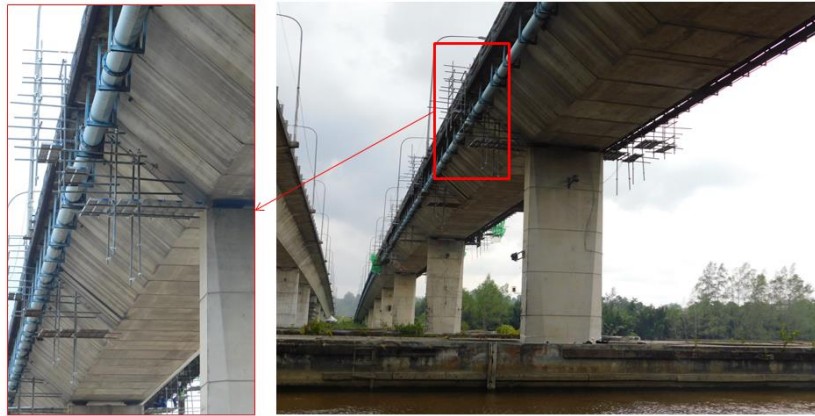
Figure 5. Working platform at a superstructure that crosses over river and high in elevation
